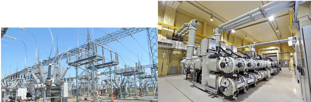
Figure 1 An outdoor (left) and an indoor (right, gas insulated) HV substation
