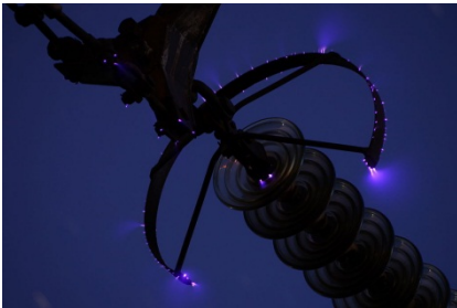
Figure 8 A view of corona discharge
