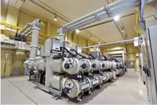
Figure 7 A Gas Insulated Substation
