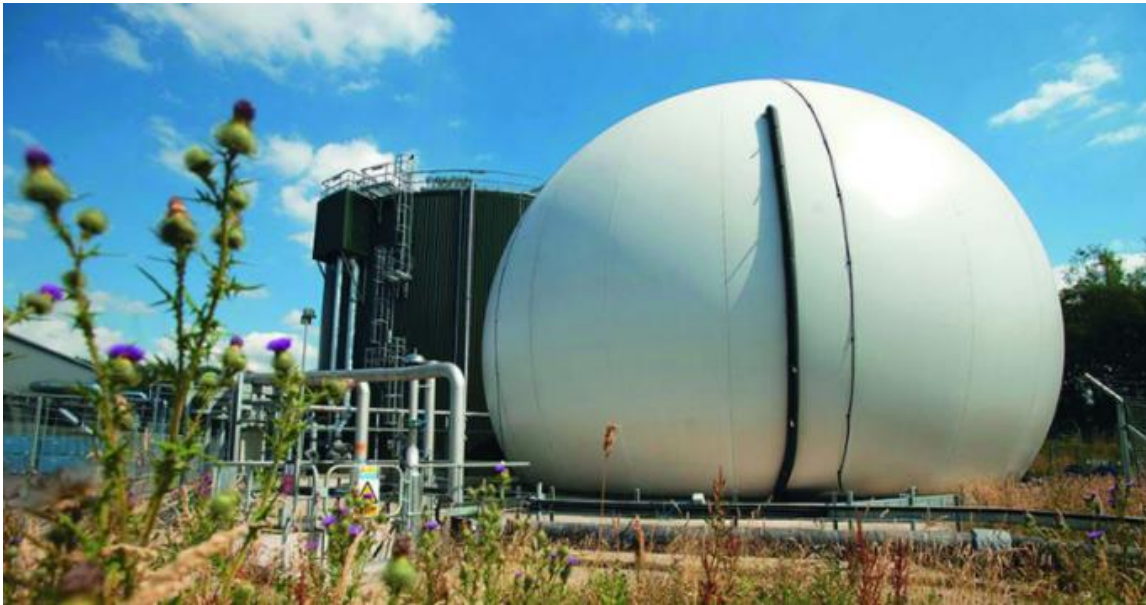
Figure 3.1: Deerdykes Bioresources Centre, Lanarkshire (Dolan, Scottish Water Horizons, 2019).
